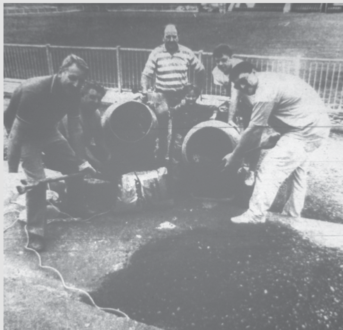
Loyal Borough fans get to grips with some concreting to complete the terracing that runs alongside the canal side of the ground. The workforce are from left: Dave Hall, John Wilson, Eddie Stevens, Stuart Swingler, Gerry Swingler and Phillip Aston. Photo: Heartland Evening News
