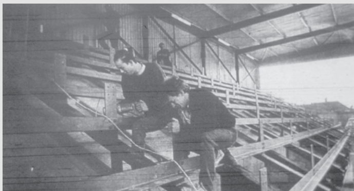
Workmen add the finishing touches to the steel supports in Borough's new stand.
